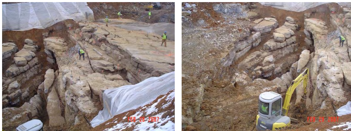
Figure H1-4. Zone of fracture concentration with gently dipping Stonehenge Limestone, Katz Law Building.
