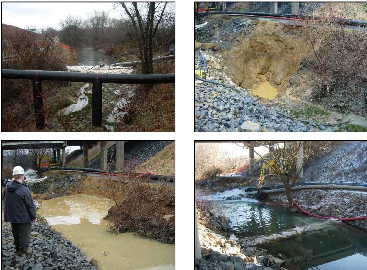
Figure H5-3. Sinkhole within Slab Cabin Run, Route 322 bridge.
